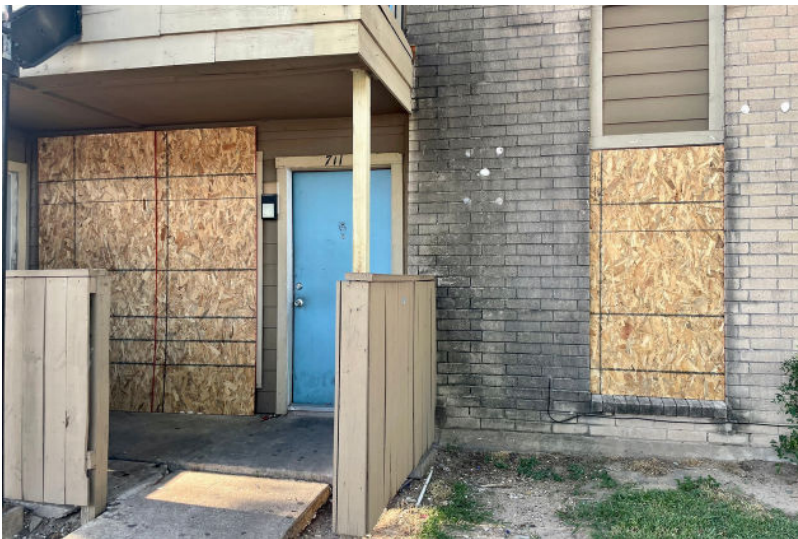
A boarded-up unit last summer at the Timber Ridge Apartments in Houston. PHOTO: MITZI ORDONEZ/TEXAS ORGANIZING PROJECT
